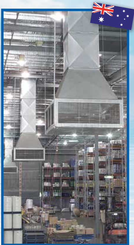
Solver Roof (Australia)
