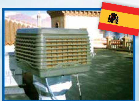
Large commercial centre, Warner Bros (Spain)
